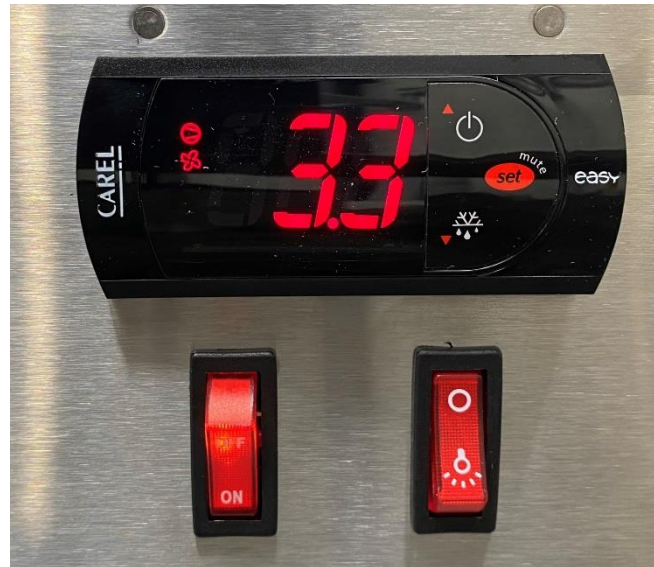
electronic controller & red toggle switches
